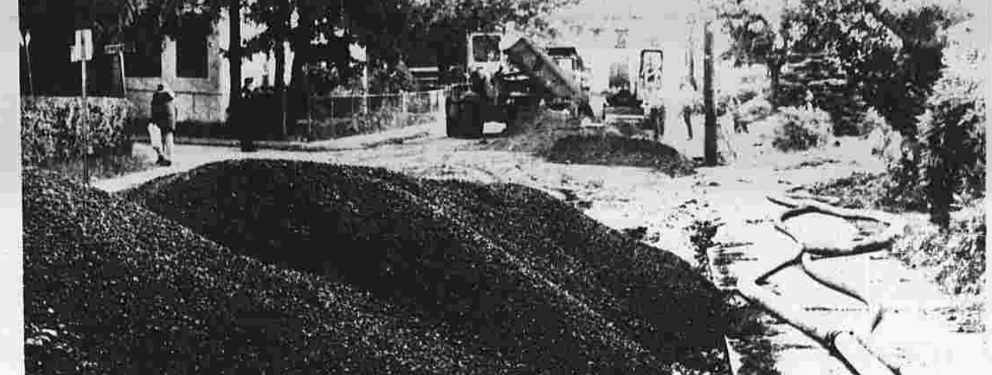
Hoses strung along Basell Street Monday carry sewage from one manhole to another as workers bypass sections of the old Porter trunk sewer line to replace it with a new one. The Glenn Construction Co. of Manchester has completed about 75 percent of the $1.6 million project and hopes to have it done by early December to avoid working in harsh weather.
